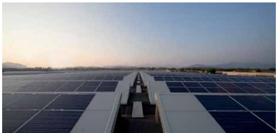
Photovoltaic roofing of the Company
