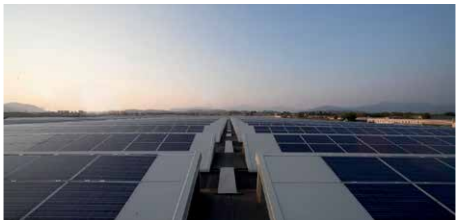
Photovoltaic roofing of the Company
